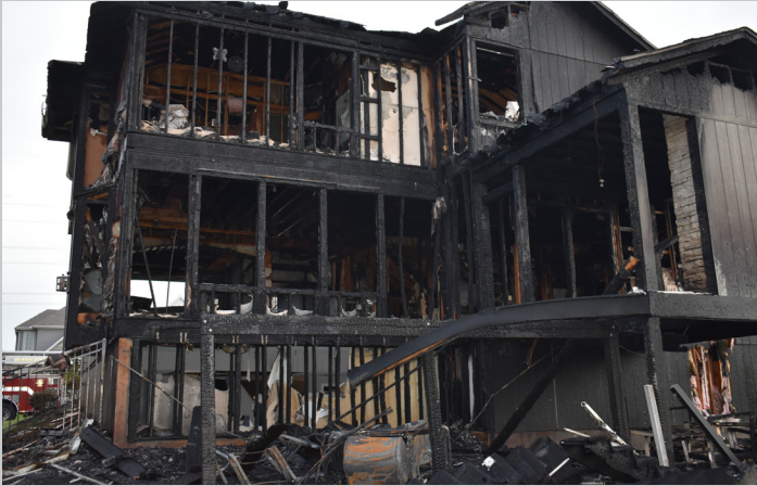
This house fire was caused by the improper disposal of ashes.
