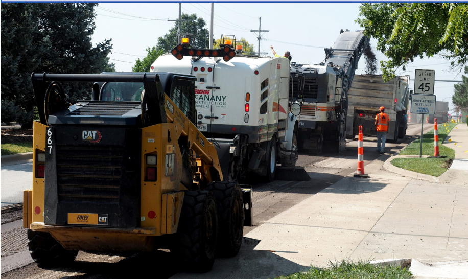
Street maintenance with mill and pavement overlay is completed on Renner Road, near the north city limit.
