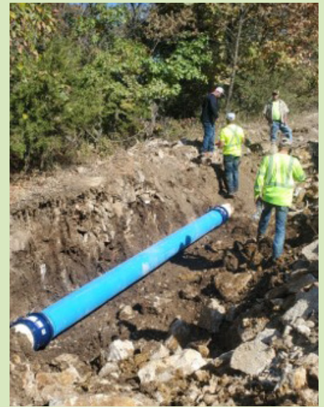
After the water main repair was made, and before it was back filled.
