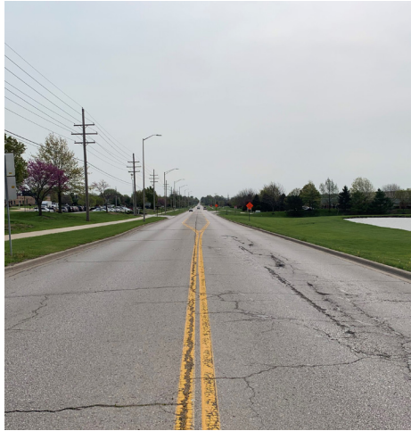
159th Street BEFORE new pavement in 2021
